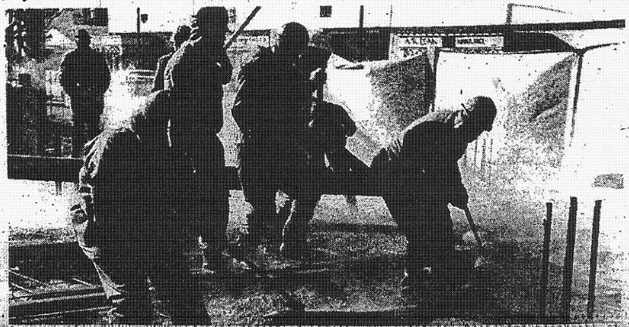
CONSTRUCTION CREW laying the foundation for a $2 million structure recently completed on Chicago's South Side for the Nation of Islam.
