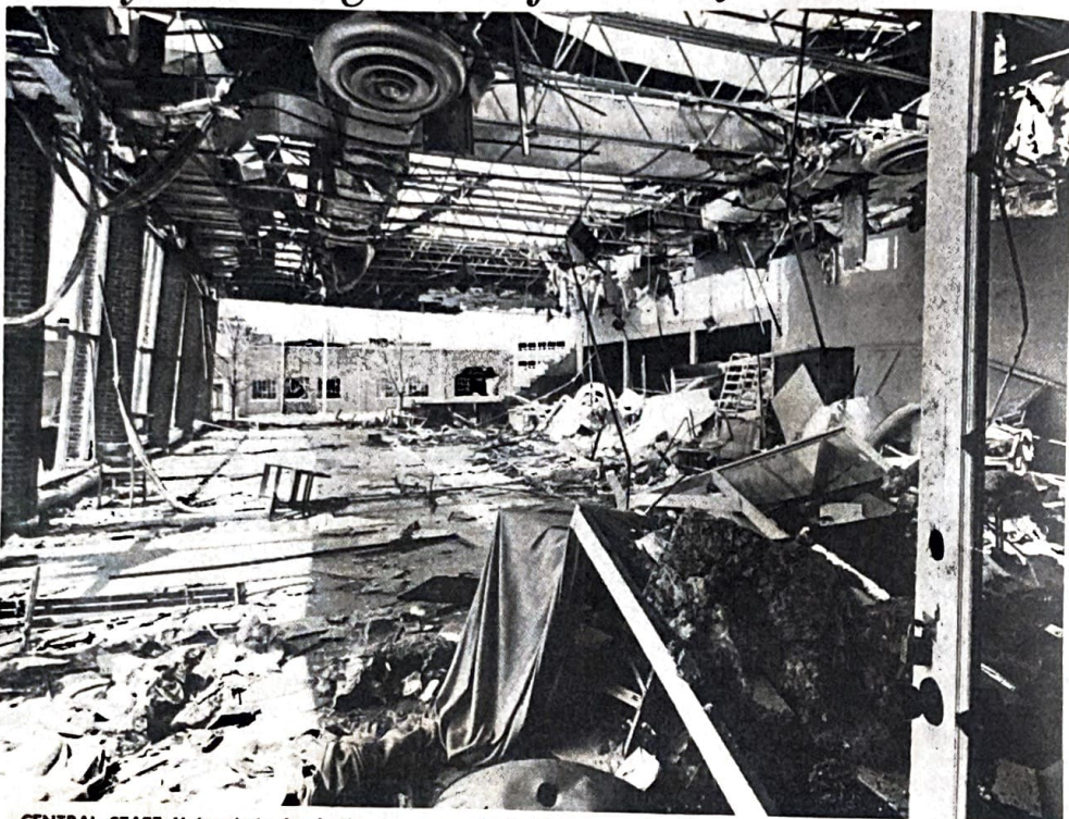
CENTRAL STATE University's Art Institute was completely blown apart by the force of last week's killer storm. (M.S. photo by Emerson Muhammad)
